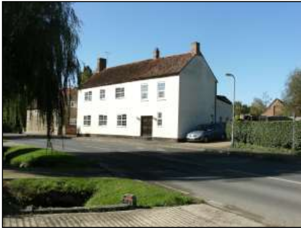
Fig.15 21 & 25 High Street. Loss of character with modern inappropriate windows and doors and render over masonry.
